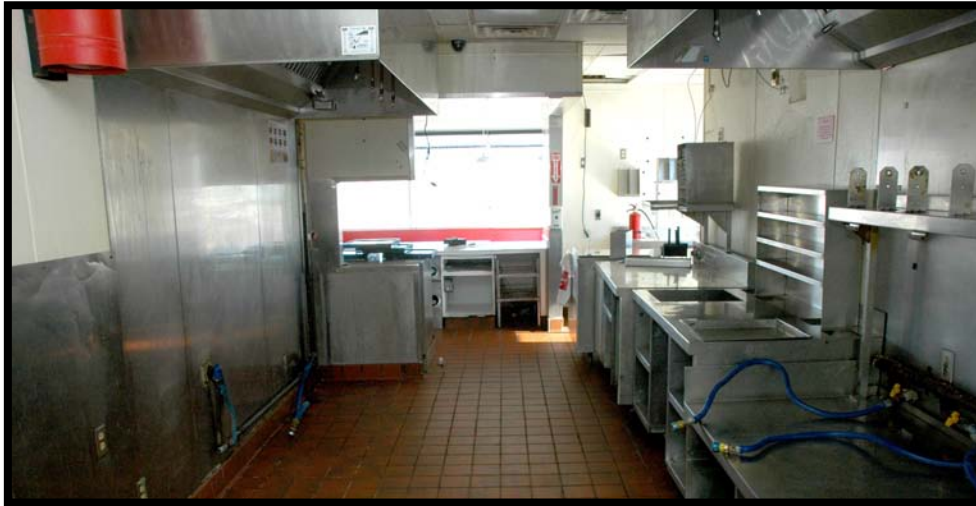
Ventilation Hood System / Fire Suppression in Place
